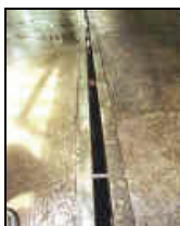
Photo 1. Dirty water generation: wash down high volume low pressure hose and drainage channel for speeding up washing after milking (Source: www.teagasc.ie )
